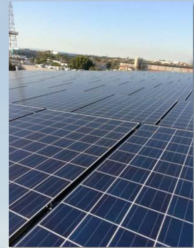
Signal Hill Facility
